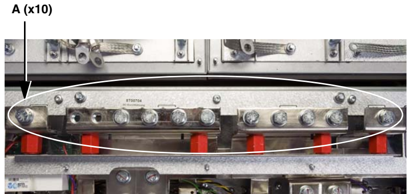
Figure 114: Bus Bar Hardware, Top
