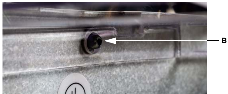
Figure 10: Power Terminal Shield Retaining Post
