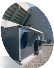
Ventilation: Air treatment plant safety/smoke extraction
