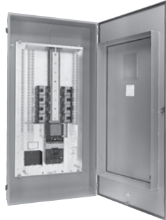
Access to Wiring Gutters
