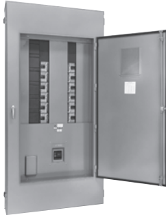
Access to Circuit Breaker Handles
