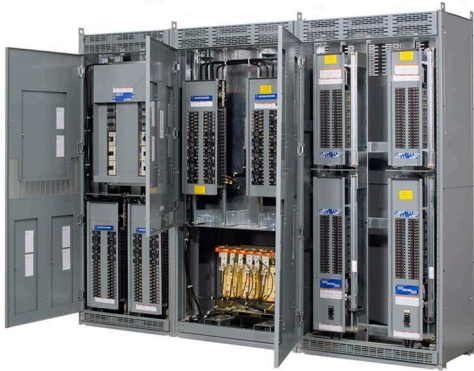
Integrated Power Center 2
