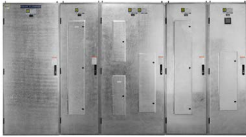
Integrated Power Center
