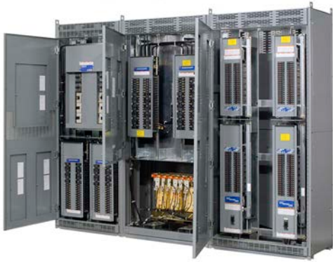
Integrated Power Center 2
