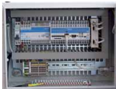
IRIO controller cabinet
