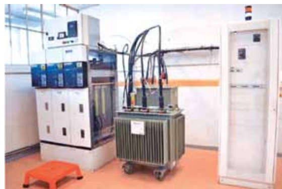
On-site cubicle + transformer + LV switchboard installation
