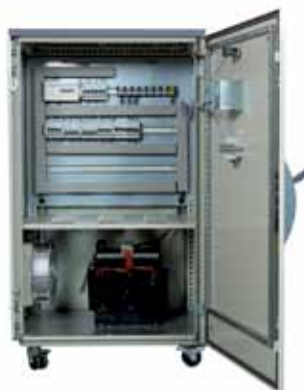
IT system cabinet
