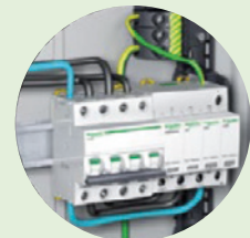
External back-up protection
