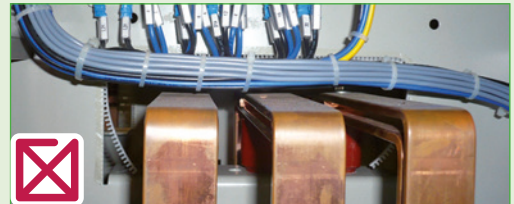
The cables are routed too close to the power busbars.
