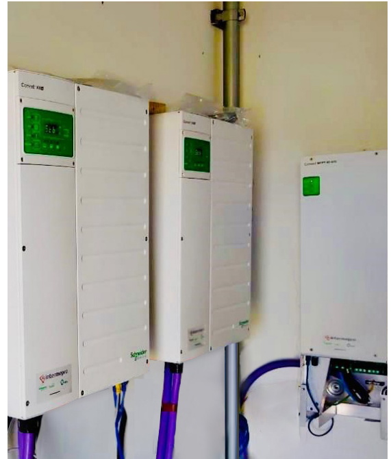
Schneider Electric Conext XW+ 7048 inverters were installed in Club Estudiantes de La Plata’s stadium
