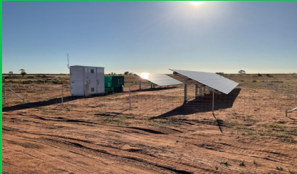
Bringing Power to Western Australia
