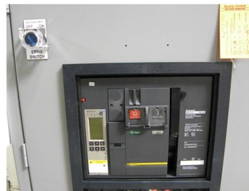
Circuit Breaker with ERMS switch
