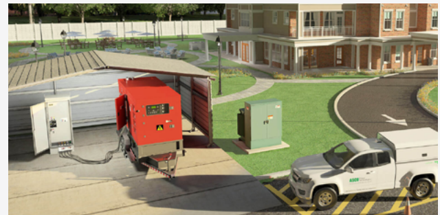
Quick Connect Panels and Manual Transfer Switches can connect small and midsize businesses to generators quickly.
