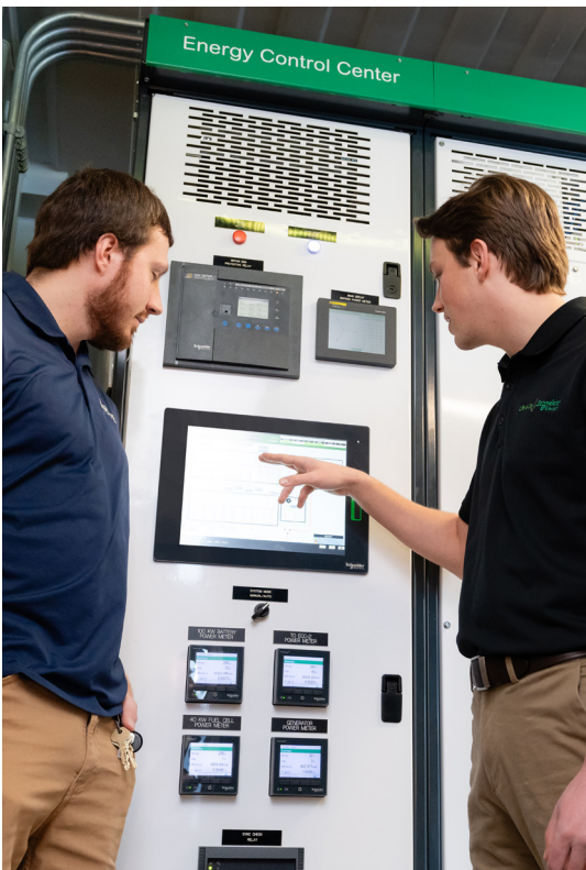
The preserve uses Energy Control Center by Schneider Electric to manage and optimize power.
