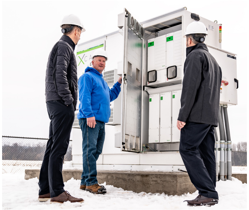
The center's Xcape microgrid solution includes Schneider power inverters, controllers, and software.
