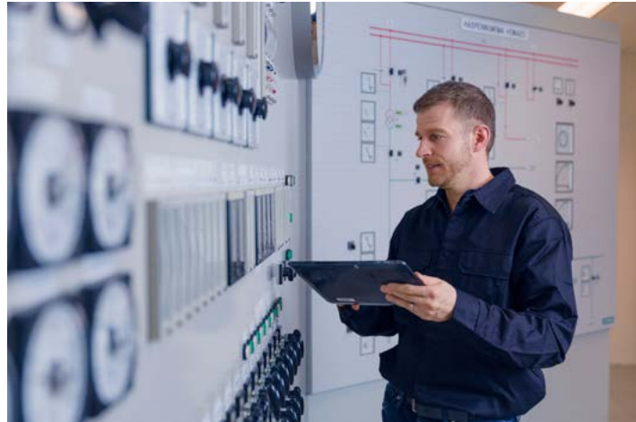
Equipment needs to be maintained regularly in order to ensure that the infrastructure operates under favorable conditions.
