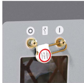
Manual switching ON of circuit breaker locked by padlock
