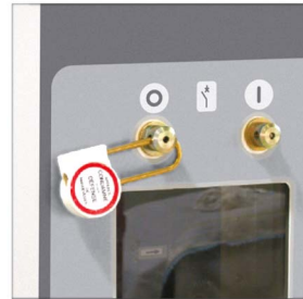
Manual switching OFF of circuit breaker locked by padlock
