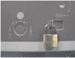
Manual racking-in of truck by padlock
