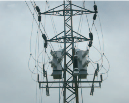
PM6 52 kV double way
