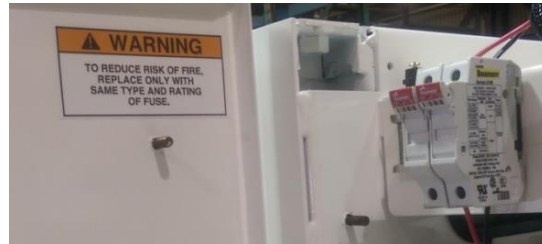
Figure 21 : Placement of fuse warning label
