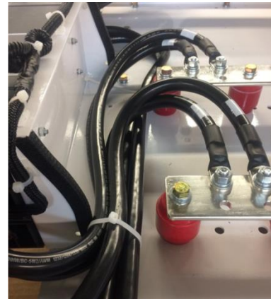
Figure 10 : Bus bar connections
