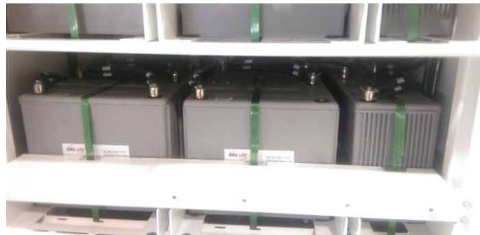
Figure 37 : Cabinet with batteries integrated
