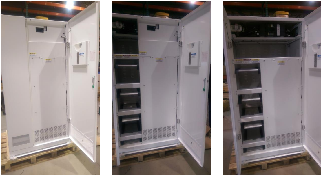
Figure 2 : Removal of dead front
