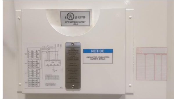
Figure 25 : Label placement on the back of the right door
