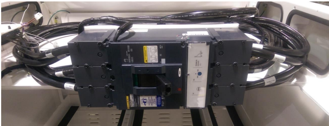
Figure 6 : Circuit breaker with trip settings to the right
