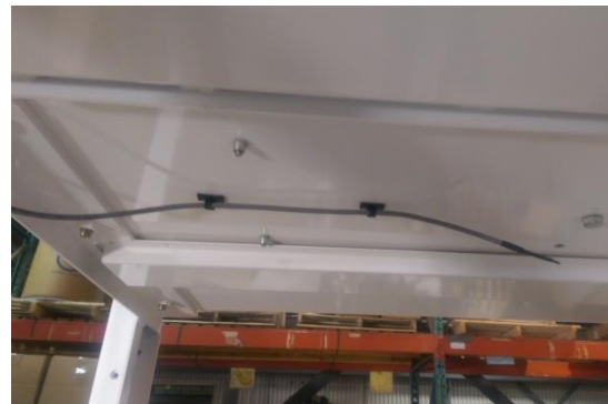
Figure 12 : Thermal sensor location
