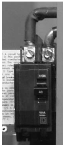
QO2100 Plug-On Circuit Breaker Installed
