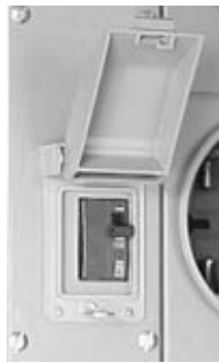
Circuit Breaker Cover, Open
